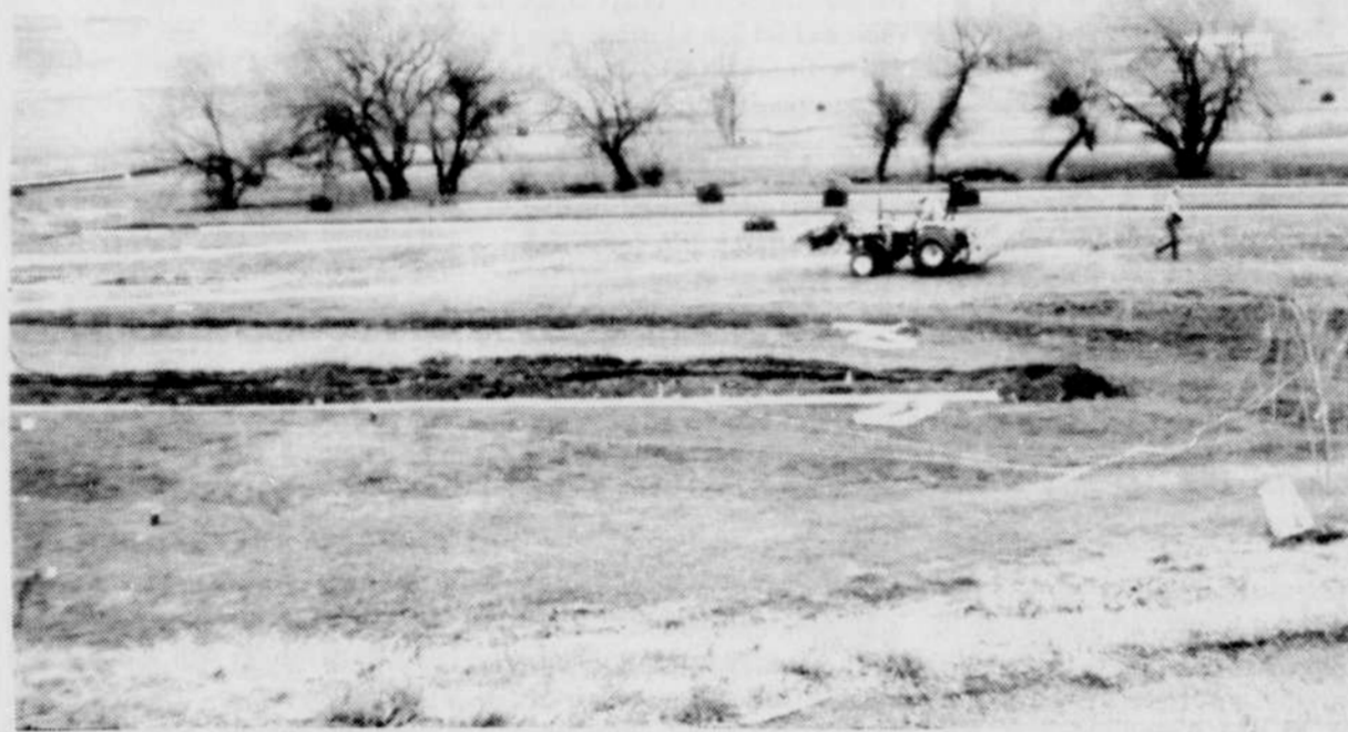
Work on the new underground irrigation system at the Willow Creek Country Club got underway recently. Treated effluent from the city's sewer system will be spread on the golf course once the system is operating.
