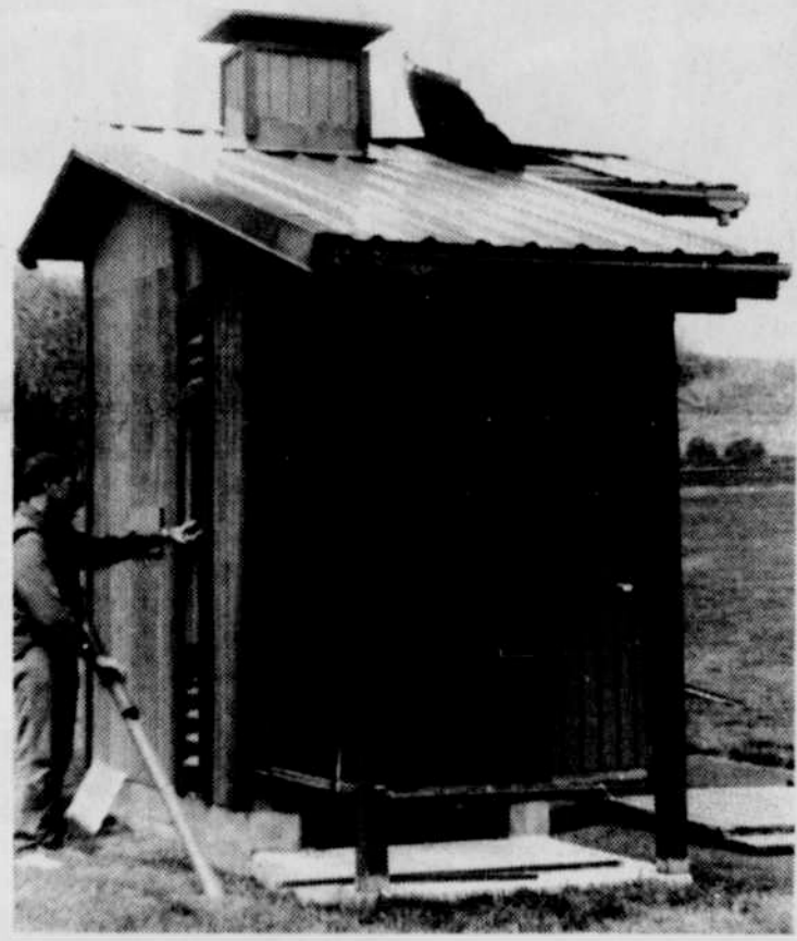
Willow Creek Park District board member Bob Kahl looks over damage to restroom
