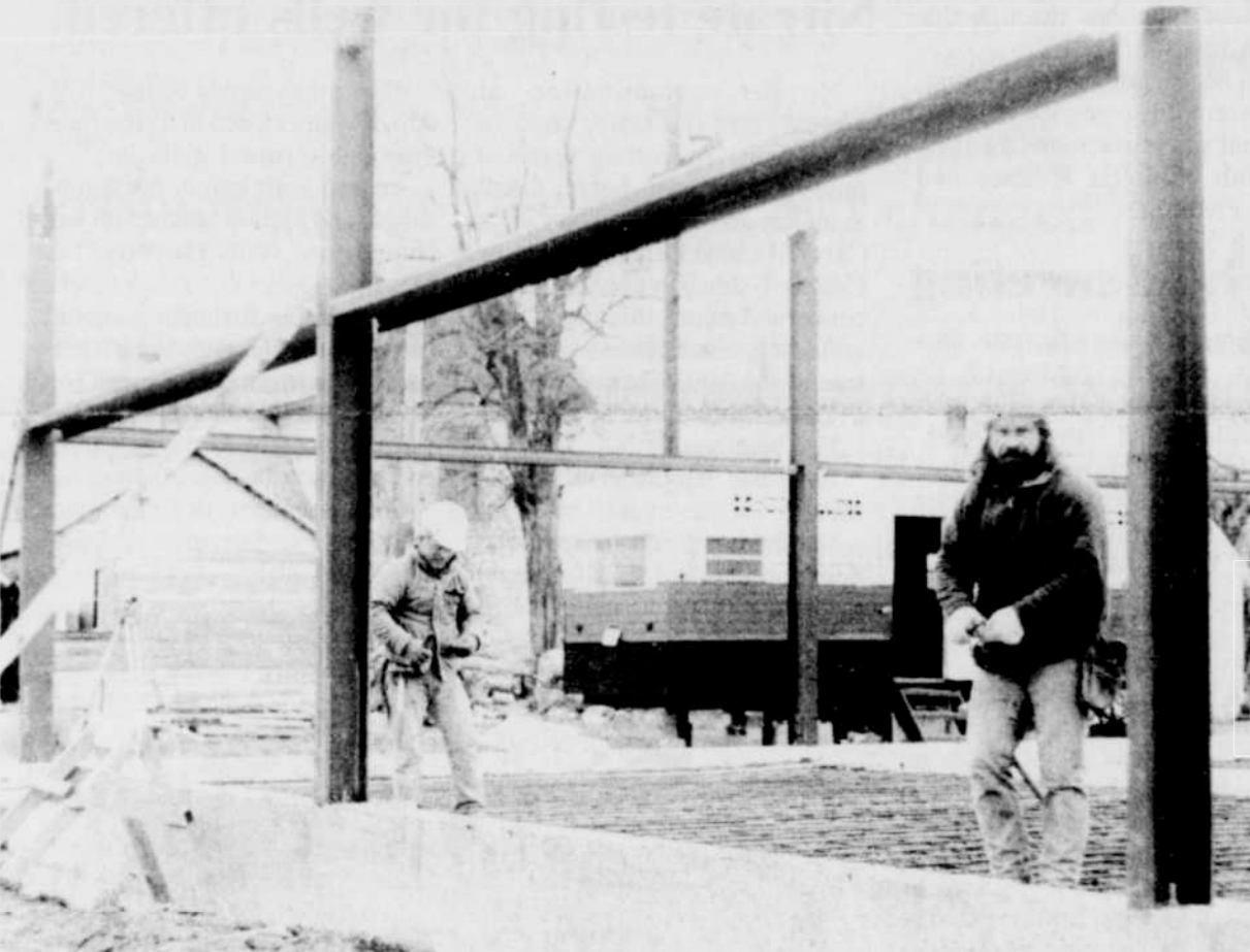
Bob Beaty (left) and Charley Dickison of McCormack construction of Pendleton, prepare site for concrete pouring.
