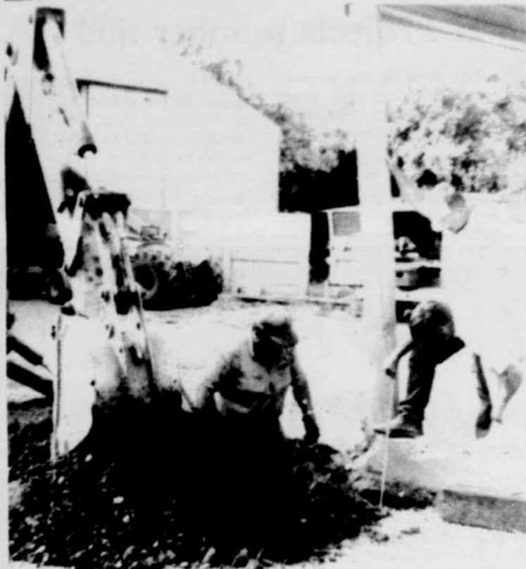
Richard Ladd (in the hole) Larry Scroggins (measuring) and Tim Coe work on stabilizing the roof on the sheep barn at the fairgrounds in preparation for fair and rodeo to be held Aug. 14-18.
