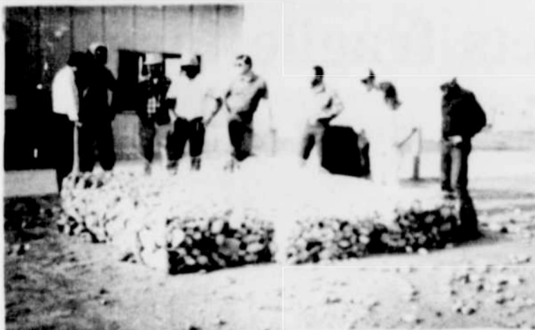
Directors view rock gabions to help alleviate wind and water erosion at the Port of Morrow Dock site.
