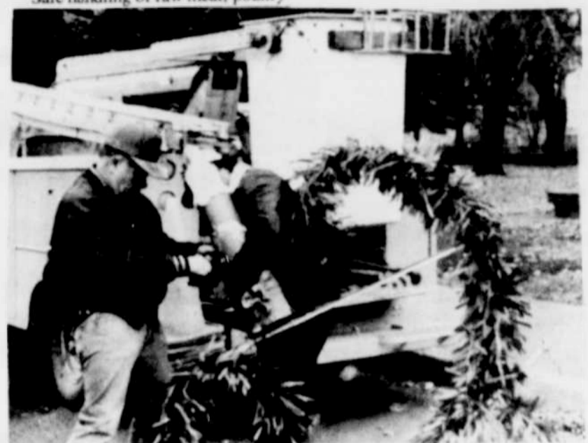
Columbia Basin Electric Co-op employee, Bud Marshall and Heppner City employee Roger Ehrmantraut help residents get into the spirit of the season by installing Christmas lights along the city streets. Columbia Basin donates its time every year.
