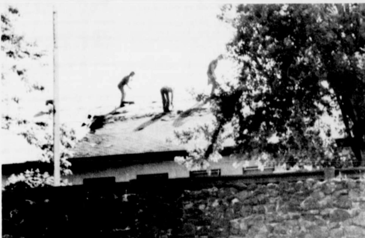
Work has started on a new roof at Pioneer Memorial Hospital. Sears has been contracted for the job. The new roofing has a 25
