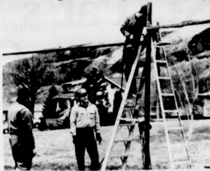
Jay Coil works on the newly installed Little League backstop up in the new field by the dam. Don Barber, Rick Paulus (L-R) along with other volunteers have spent a lot of time working on this project
