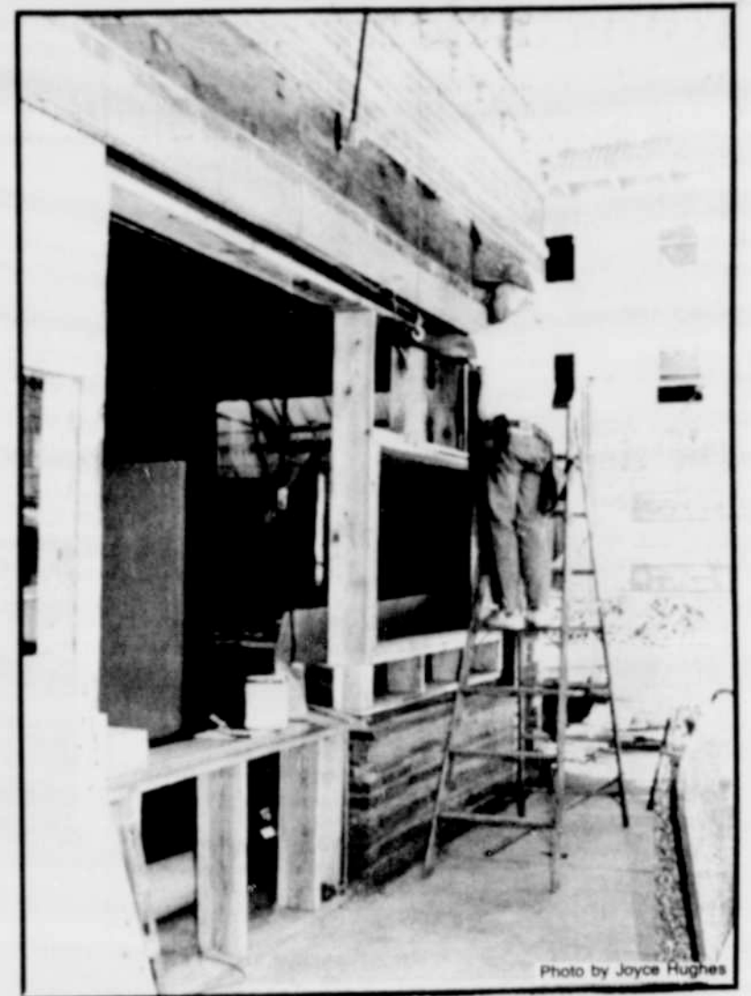
The Wagon Wheel Cafe was getting a new look last week. Chuck Marquardt is doing the work on the building which is just about complete.
