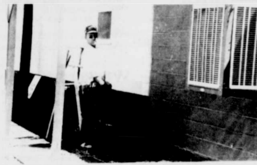
Ed Struthers is doing a lot of painting on the fair buildings this week. The structures are receiving a coat of pearl gray paint in preparation for fair week which begins August 17-21.
