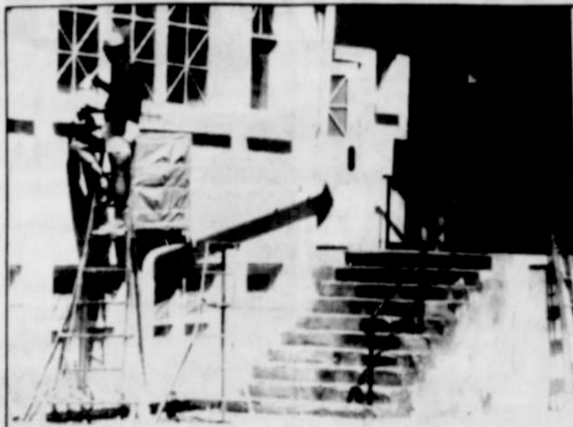
The First Christian Church in Heppner got a face lift recently. The church was sand blasted and repainted by A Sharp Painter from Pendleton. The job was finished in a week.
