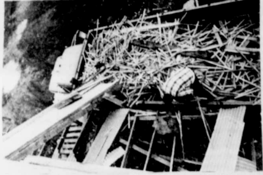
Bob Isted is loading scrap lumber from the inside of the hotel onto a truck at the community workday.
