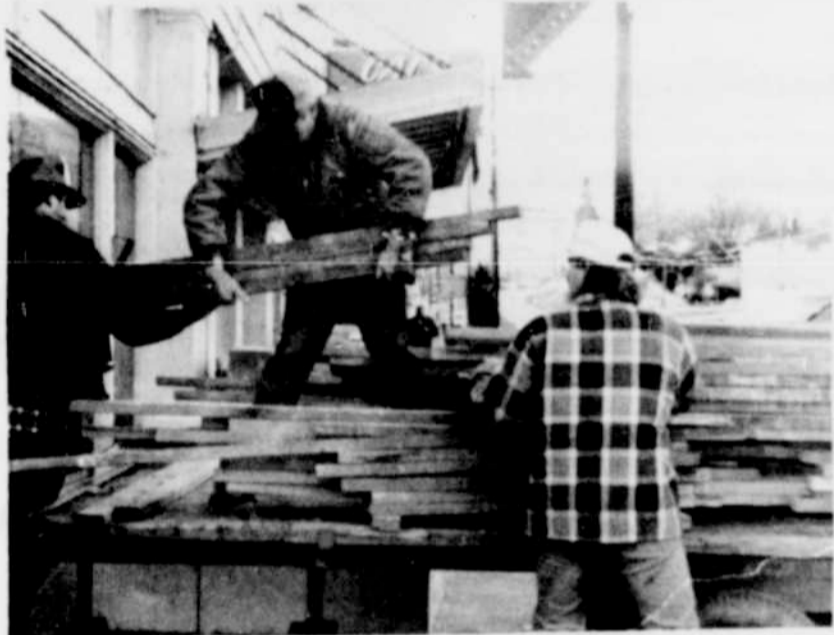
Robin Metz (l) Fred Lundin, (center) and Clint Carlson (r) are loading scrap lumber from the hotel project. A good crowd showed up for the community work day.
