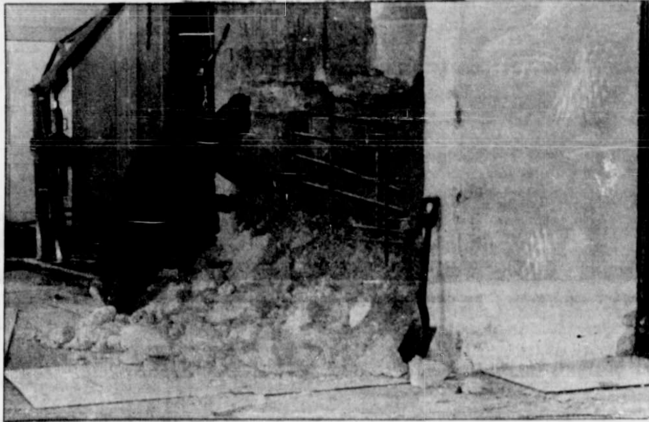
Wilbur Jackson is using a jack hammer to take the safe out of the old Heppner Hotel. Work started on the renovation of the hotel this week.
