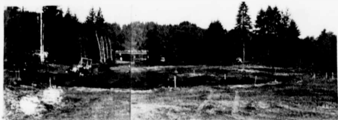
Operating engineers training school, which has agreed to do work on construction of the Willow Creek Park, is shown here working on a little league park at Reedsport, Oregon.
