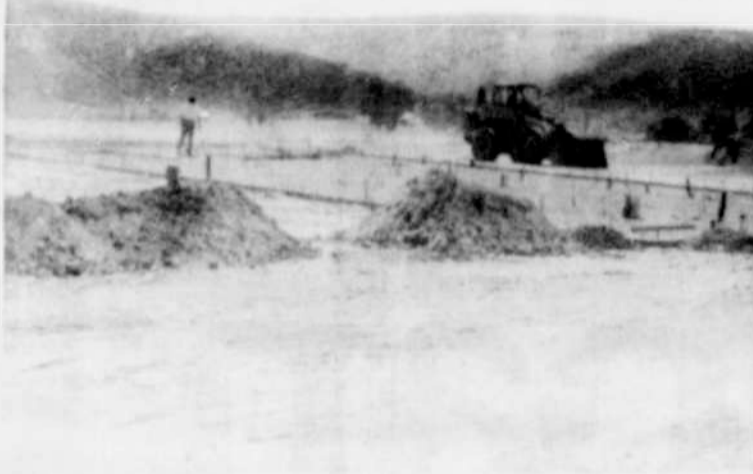
Construction is underway at the site of the new Mormon Church building in Lexington. Groundbreaking ceremonies were held June 21 with the church's state president Allan Alder and Morrow County Judge Don McElligott present. The white brick building is expected to be completed by late October or early November at which time an open house for the public will be held.
