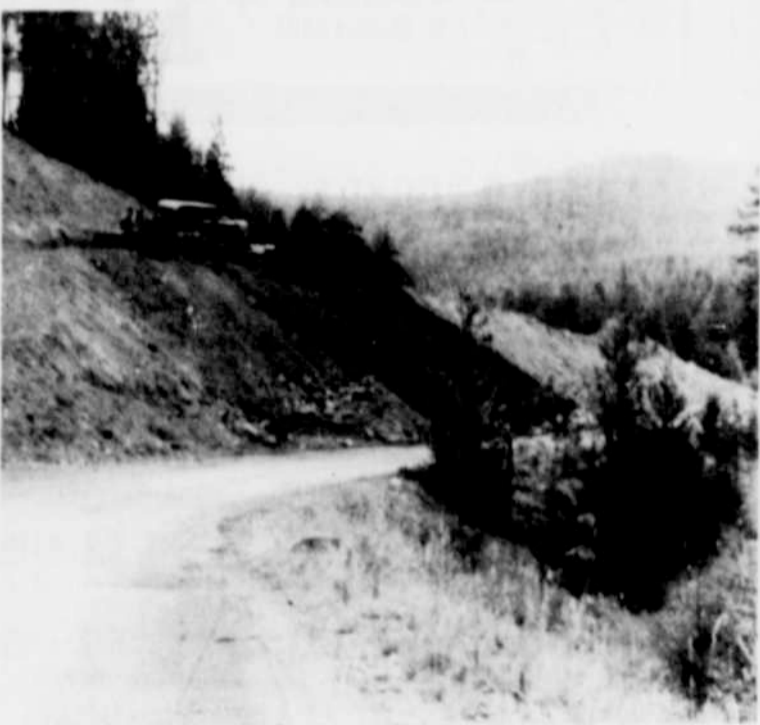
Dozer makes cut in hillside for new roadbed on Willow Creek Road
