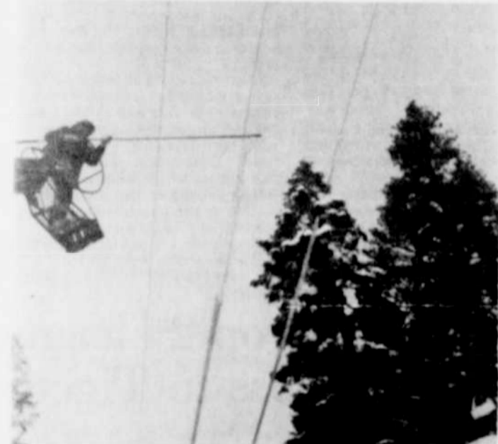
Removing ice from lines near Cutstorth Park
