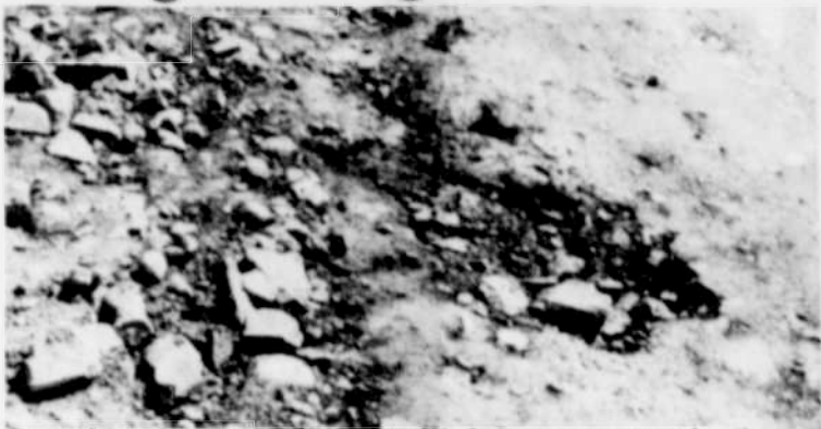
The surface of the sub-grade road bed before it was covered with sub-base rock.
