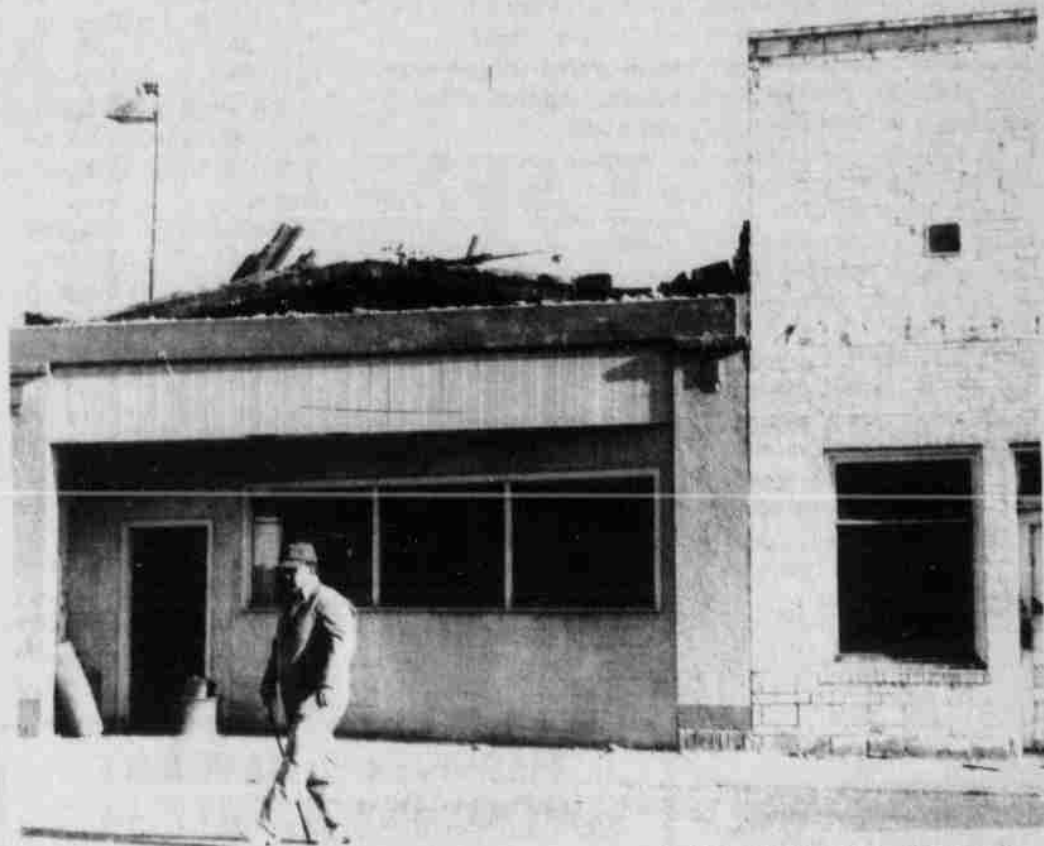
Dave Barnett stands in front of the old Stefani's Restaurant Building (left) and the old I.O.O.F. hall on Main Street in Ione. Both buildings are being torn down.
