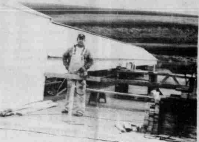
Mel Piper modified several barn designs to come up with the result he has built here.
