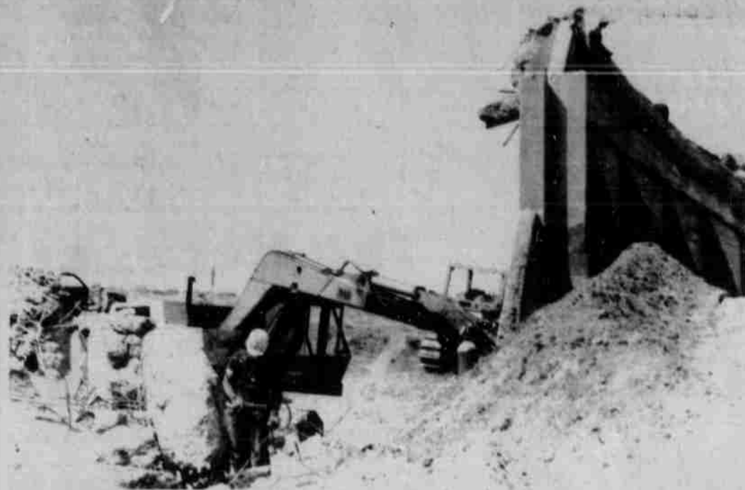
Workers remove debris from an existing structure that was in the way of the new overpass west of Boardman.
