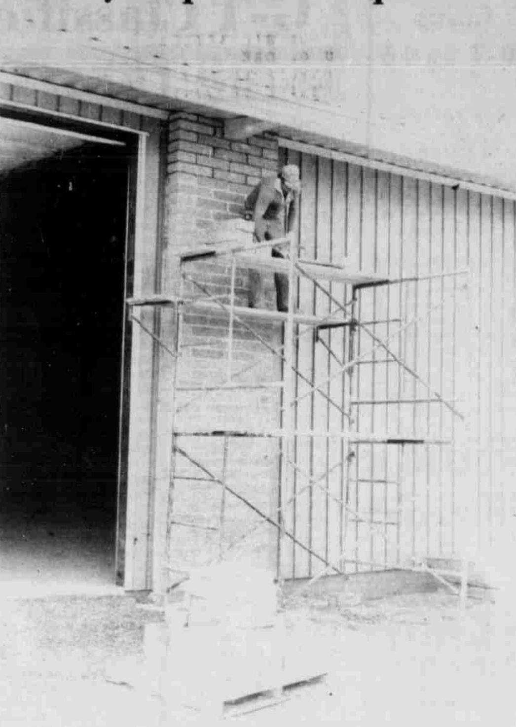
Workmen put finishing touches on new county shop building in Lexington. The new shop will be completed and ready to move into in about three to four weeks.
