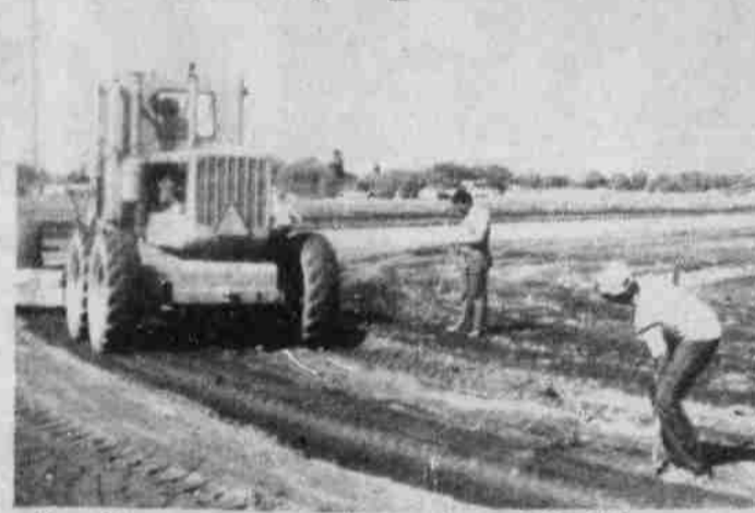
Jim Key operates a grader while Vic Marcher (L) and Jeff Wenholz help prepare a new athletic field at Columbia Junior High
