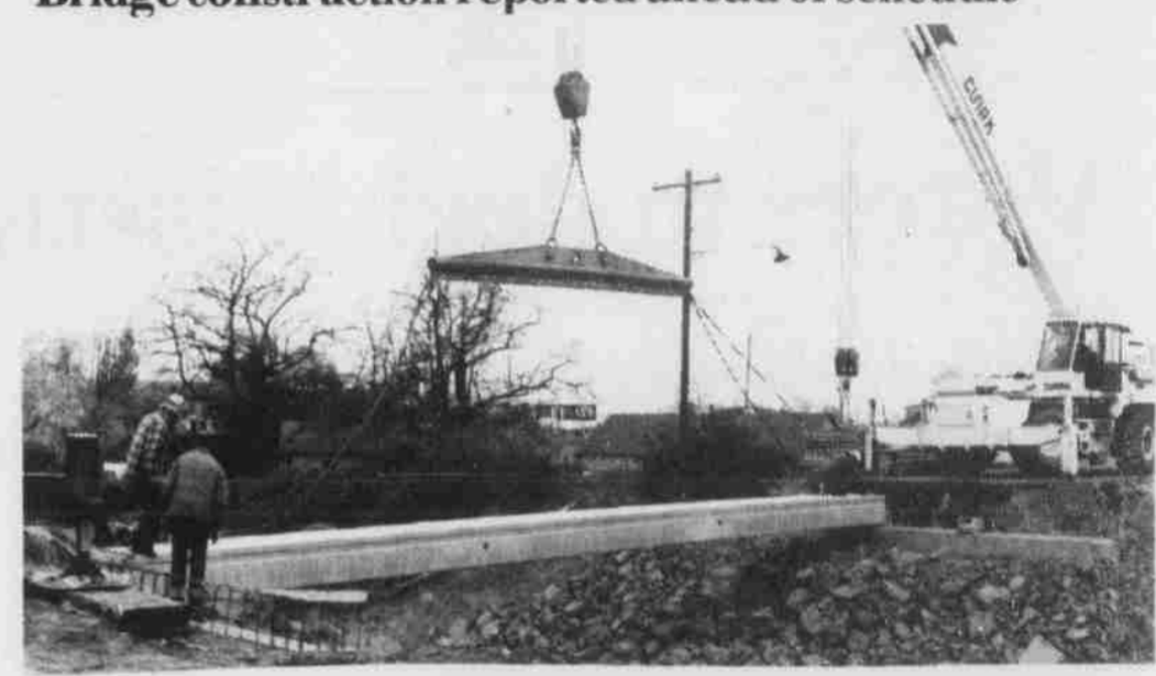
Workmen lower cement span during construction of new bridge on Arcade Street in Lexington Monday morning. The old wooden bridge was torn out and the new bridge is being built. Construction on the $125,324 bridge is reported to be ahead of schedule.
