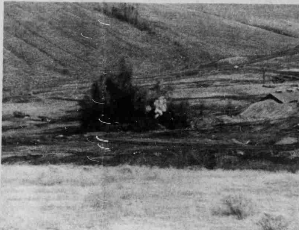
Eucon Corp. has begun blasting at dam site. Rock will be crushed and used with cement for dam construction.
