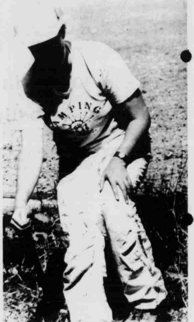
Annie Johnston, Forest Service recreation guard at Bull Prairie, digs post holes for traffic barrier posts.
