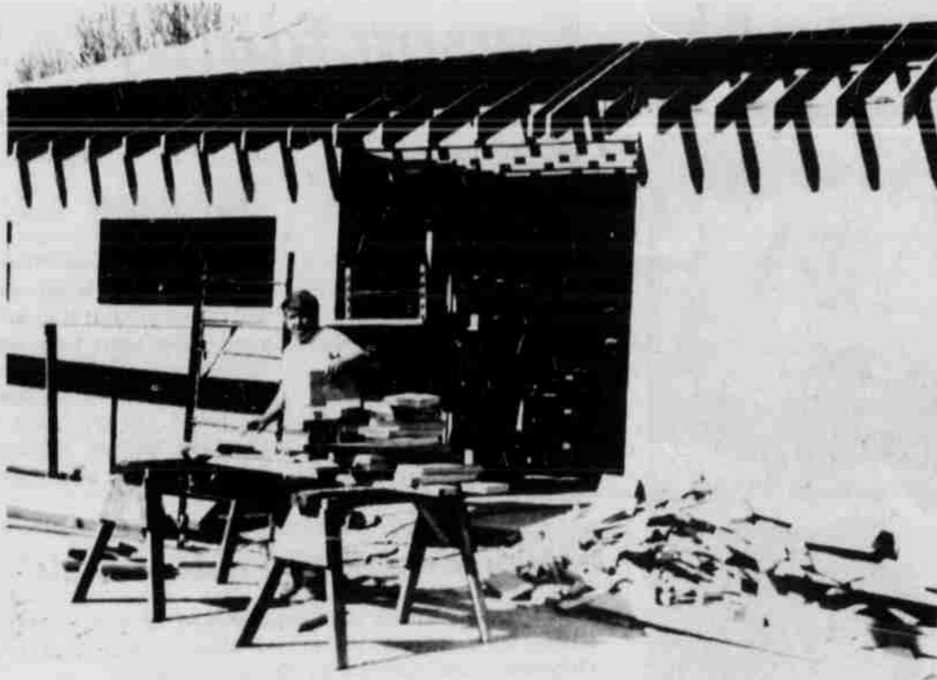
Work on the Pioneer Memorial Hospital expansion project is scheduled to be done by July 18.
