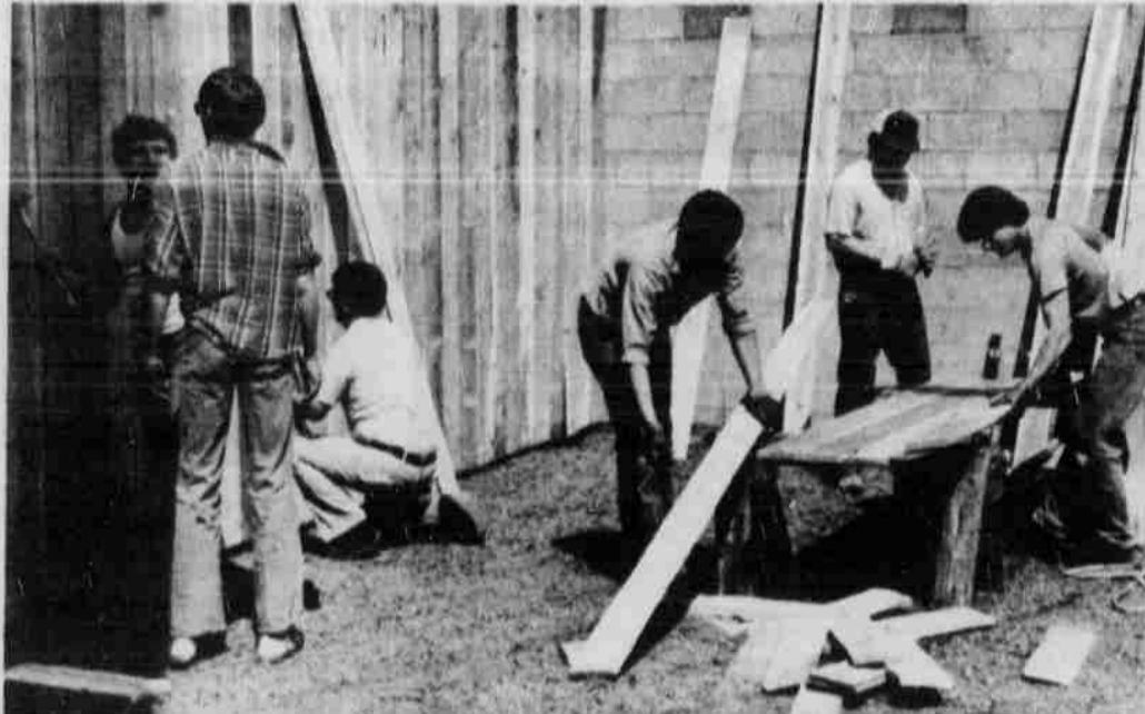
Members of the Heppner Lions Club were busy Saturday erecting a fence at the new little park they are developing on Main Street. Next they will place a community bulletin board and a couple of benches where people may sit and watch the passing traffic.
