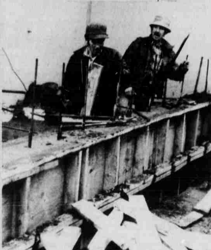
Workers on the Pioneer Memorial Hospital expansion project continue working despite the crazy spring weather the county has had lately.
