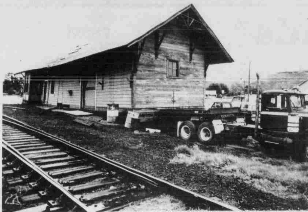
The old Ione Railroad Depot was moved from its familiar location close to the Union Pacific railroad tracks recently by Mr. and Mrs. Marvin Peterson who plan to convert the early structure into a home above Horeshoe Bend 6 miles away. (Birdine Tullis Photo)
