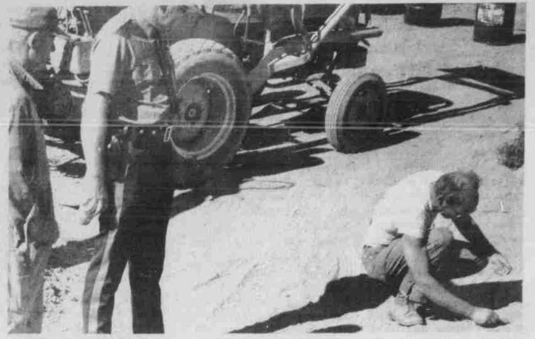
Wayne Gray touches a match to a stick of dynamite—part of five cases—unearthed as he and other workers were digging a water line trench to the new Ione well. At the direction of Oregon State Police the hot stuff was burned after having laid underground since the early 1900's.
