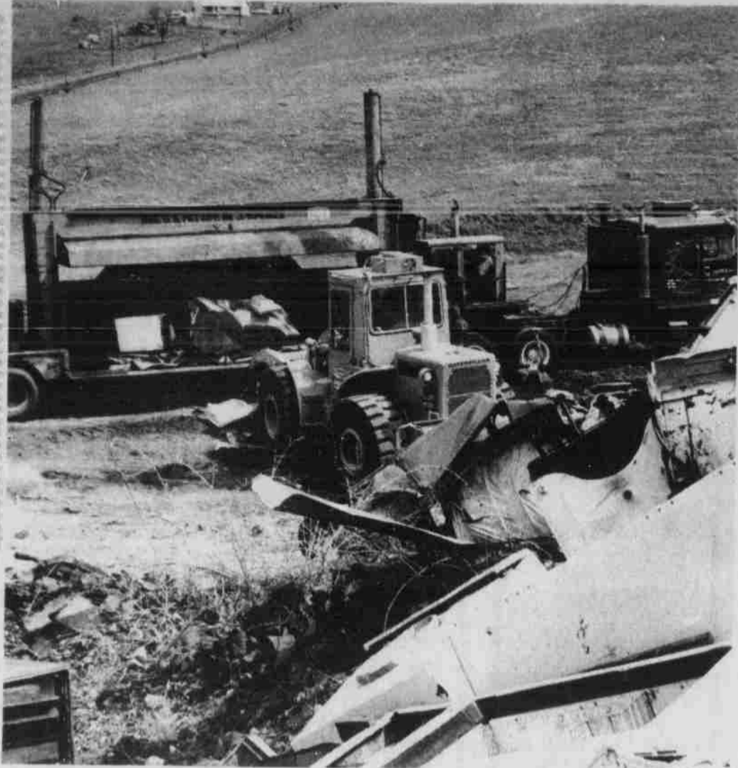
The Crusher goes to work smashing car bodies and metal items at the old city dump. The 50,000 pound unit can develop 140 tons of crushing pressure. The cleanup of the old city dump involved about 10 days of work, not counting earlier work by volunteers. Heppner now uses the county landfill. Also shown is a 950 articulating caterpillar wheel loader with crisp grapplers.
