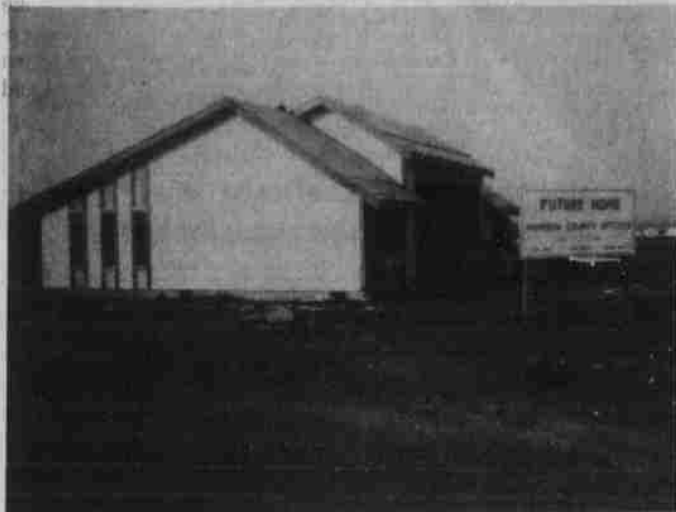
Framing has been completed on the new Morrow County Offices building at Irrigon and occupancy is expected about March 1. The new office building is located at the corner of North Main and Second Street.
