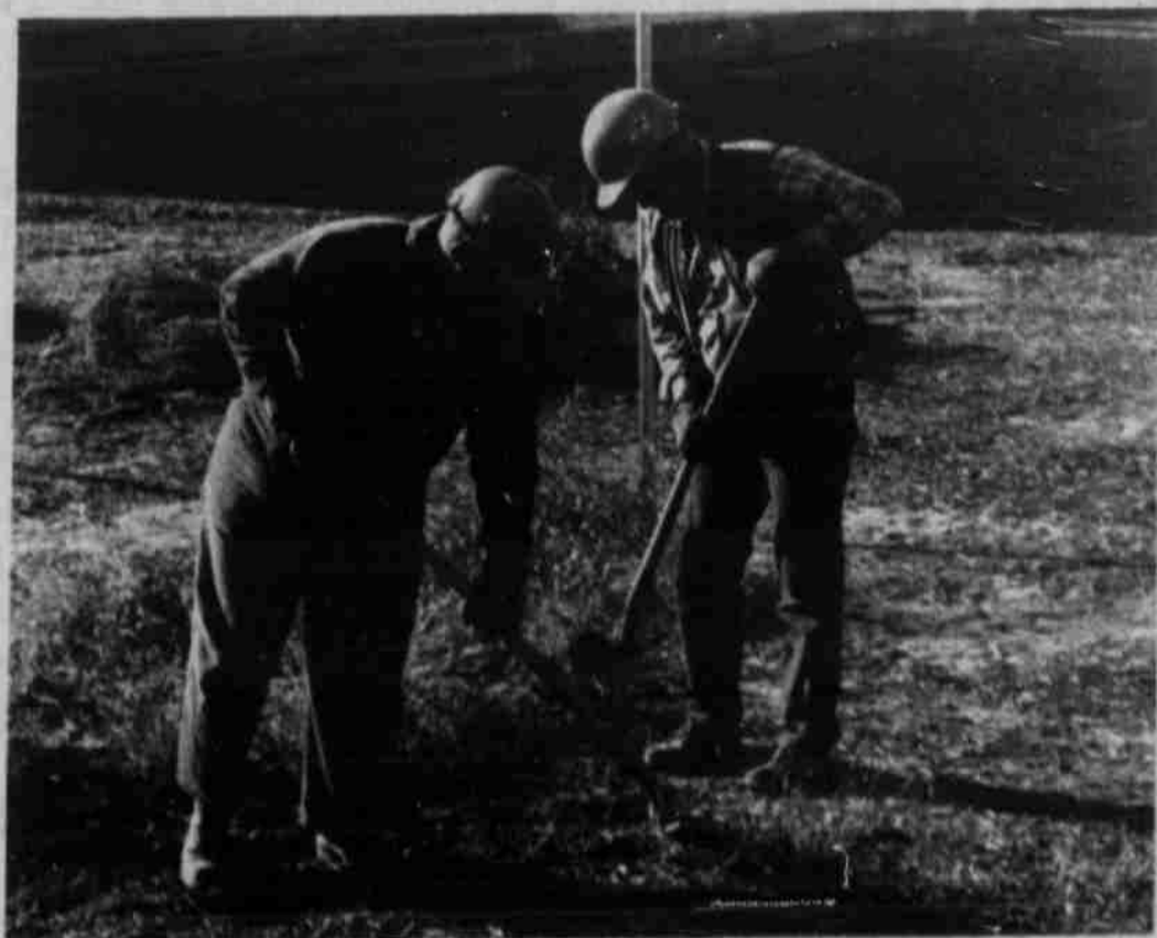
Workers clear roadsides. Fence behind will put Kinzua production on west side of road completely. Trucks won't have to cross highway.
