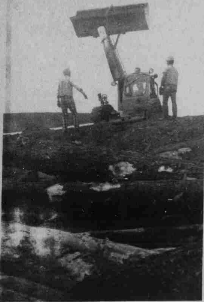
State highway employees replace posts along turn of highway towards Condon. truck missed turn
