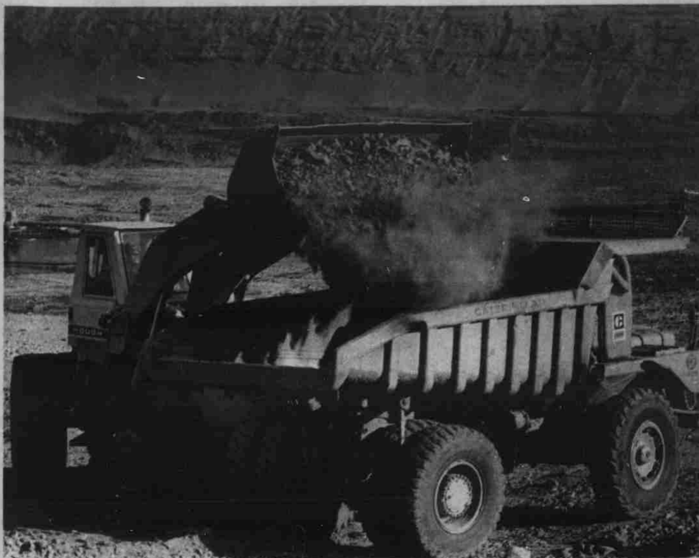
A couple Kiewit rigs turn bleak landscape into energy producing coal-fire plant.
