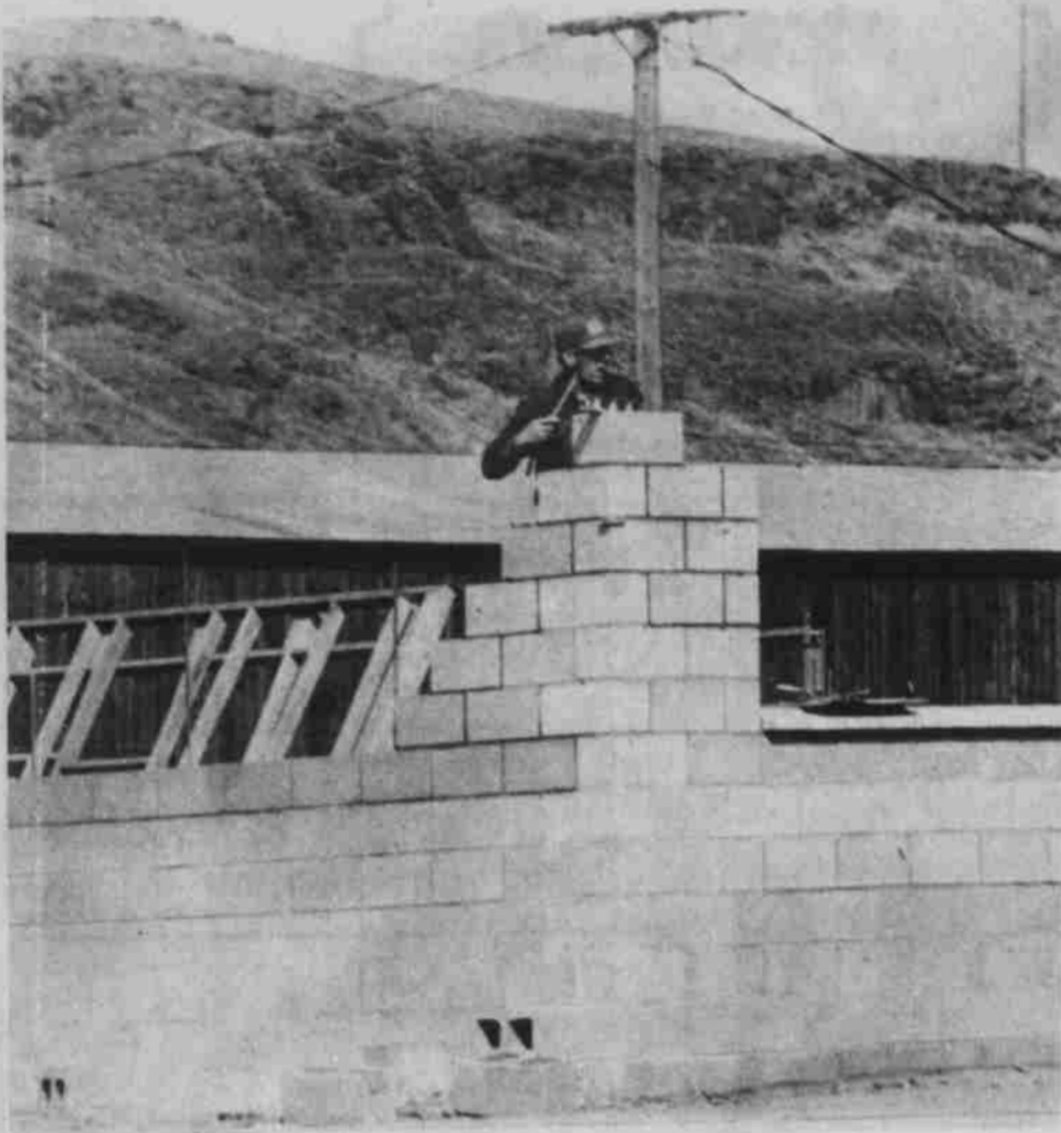
The Office on Main St., lone is being rebuilt. Contractor Cliff Aldrich adjusts his string line before adding more concrete blocks.
