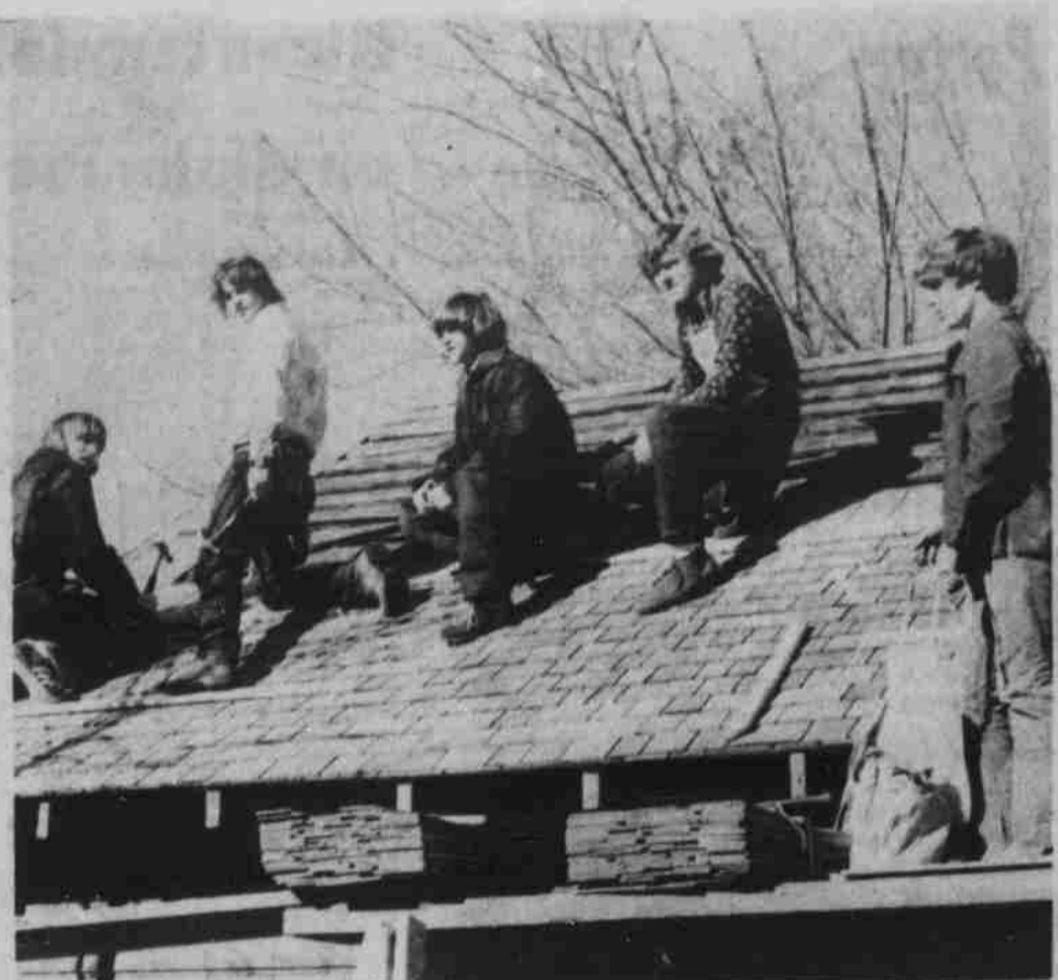
Students of Heppner High School in Construction Class 2 are putting wooden shingles on the roof of the Democrat Gulch schoolhouse. The students are interested in construction and this is part of their training program. The instructor is Ed Heimstra. From the left, Rob Eckman, Mike Orwick, Doug Harris, Dave Brandhagen and John McLean.
