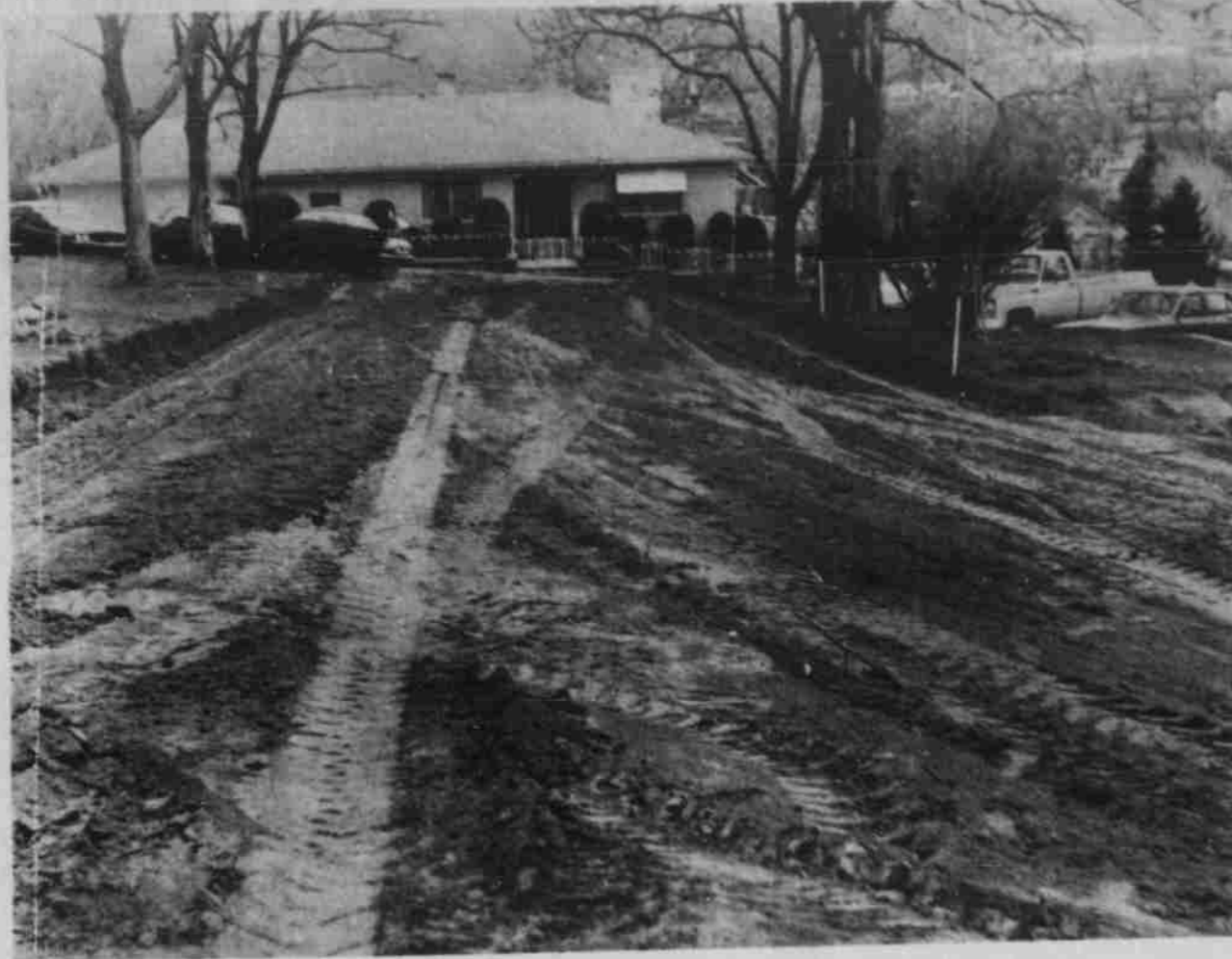
With more and more people doing business at the Morrow County Court House, there has become less and less space for parking, so the county decided to do something about it. Here a new roadway has been cut east of the courthouse, which will run through from the existing parking lot to Cannon St. The new road will allow both parallel and diagonal parking to alleviate the present parking problem. Curbing will be installed on each side prior to paving the roadway.
