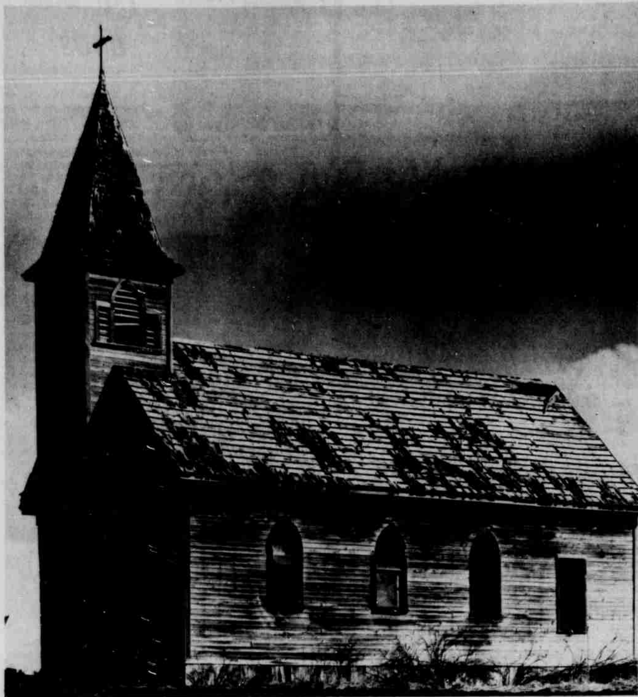
Cold spring winds now whistle through the loose shingles of this once stately pioneer church in Eastern Oregon, a greying reminder of days gone by.
