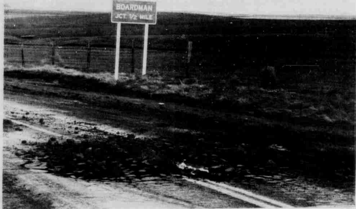
Torn up roadbed on Highway 207.
