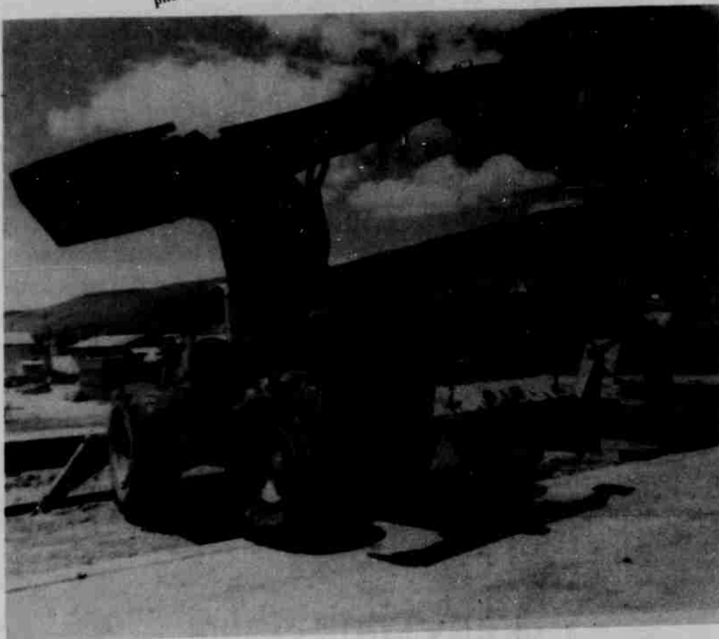
This portable boom is used by the Kinzua Corporation for various tasks. Here the boom is being used to remove the concrete forms from a newly poured retaining wall.
