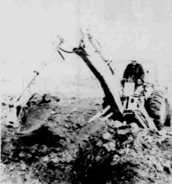
Wilson Construction crews are shown at work on the 69 kv Ruggs line for Columbia Basin Electric Coop. As pictured, most of the hole digging is "rock."
