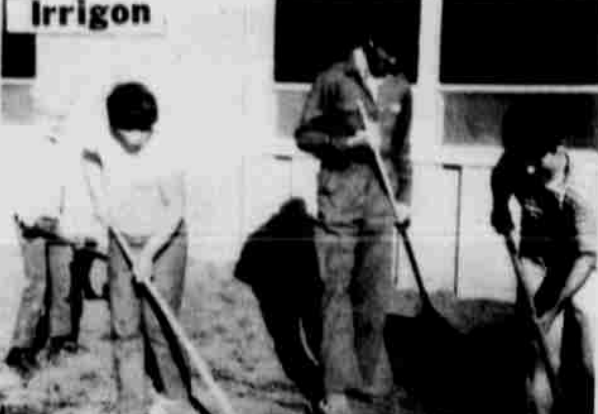
These busy 4-H'ers helped prepare the ground for lawn seed on Sat. They are 4 of the 12 Community Pride Club members who installed a sprinkler system and lawn at the Fire Station. From left to right, Jimmy Peck of Boardman Lerry Wilson, Dave Richards and Donald Richards, Irrigon. Photo by F. Wilson
