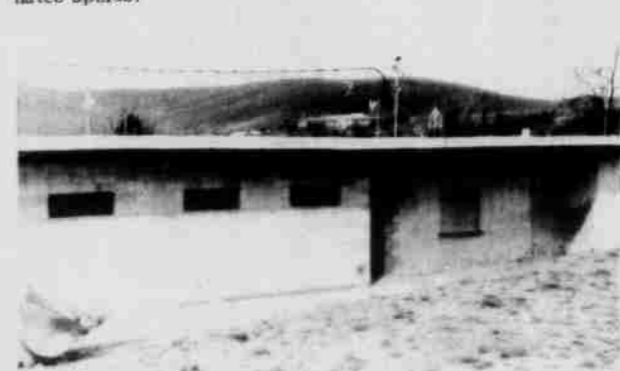
Progress is being made to get the Swimming pool ready for the summer swimming season. The outside walls have been replaced as good as new. On the right of the picture, the waterline of the May 1971 flood is still discernible.
