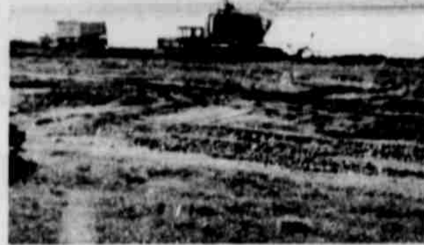
IRRIGON PARK MARINA enlargement has started. Besides a boat basin, there will be a fine picnic area provided.
