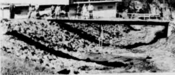
About mid-stream, the second crane is stretched out to take a hold of the beam.
