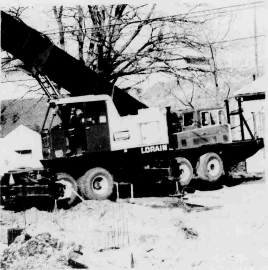
The crane on the south bank is not equal to the demands of the big beam. The hind wheels come off the ground a foot. Something else has to be tried.
