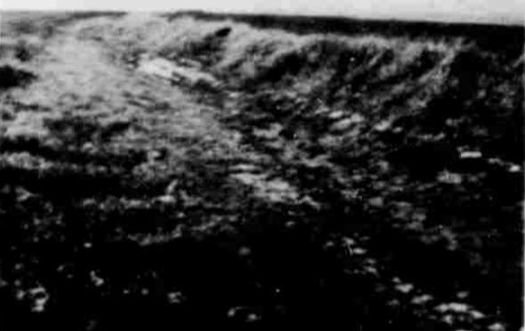
A diversion ditch on Marcel Jones farm, Marcel, 1971 Conservation Man of the Year, has over 50,000 feet of diversions installed.
