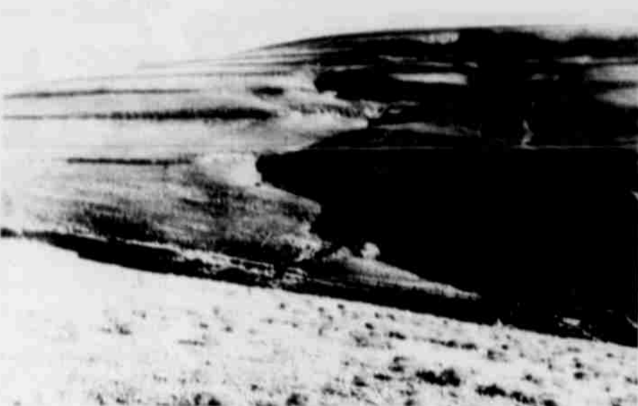
Diversion construction on Shobe Canyon drop. Slopes are near 200 feet and on slopes up to 20 percent. This field has 11 diversions from top to bottom.
