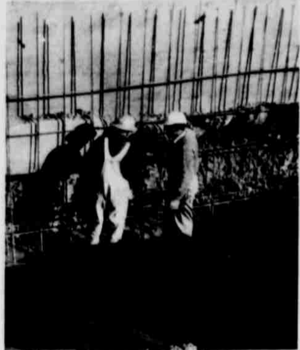
TWO MEN IN A HOLE!! tying reinforcement steel for the footings on the new Chase St. bridge. The initial construction of the two bridges over Shobe on Main St. and Chase St. got underway last week.
